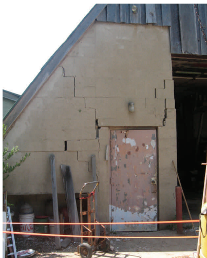
damage to cinderblock walls of MT
